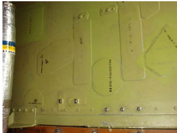
Figure 5-4. Typical Avionics Bay Honeycomb Panel Damages.
