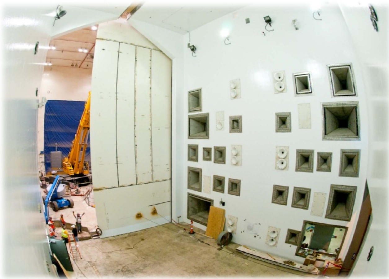
Figure 7.—Construction photo with view of the RATF chamber and horn wall taken during the installation of the main sliding door.
