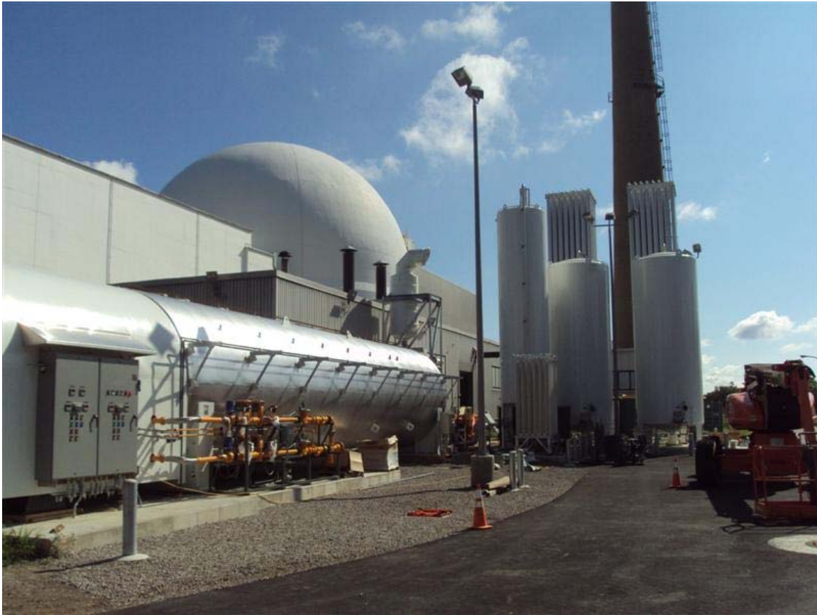
Figure 8.—Construction photo showing the RATF nitrogen generation system, including the water-bath vaporizer and the liquid nitrogen tanks and vaporizers.
