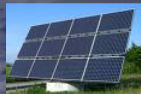
Ground PV Solar Array
