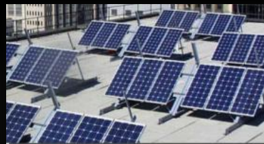
Rooftop PV Solar
