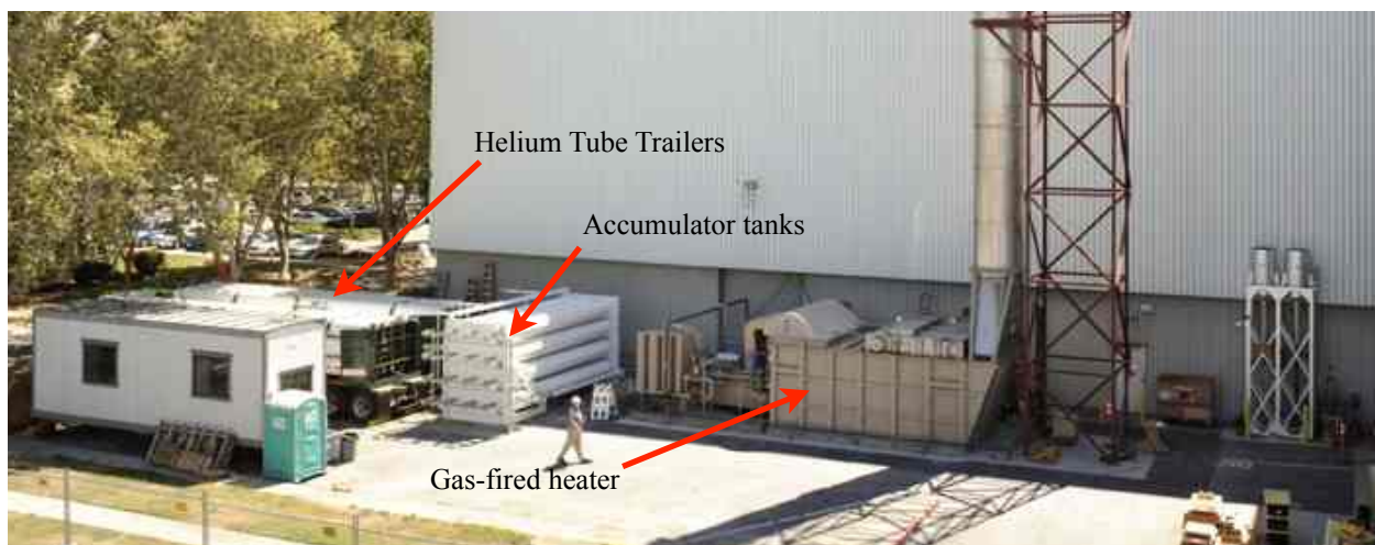
Figure 21. Helium supply system for Abort Motor plume aeroacoustics test in 11x11-Foot Transonic Wind Tunnel.
