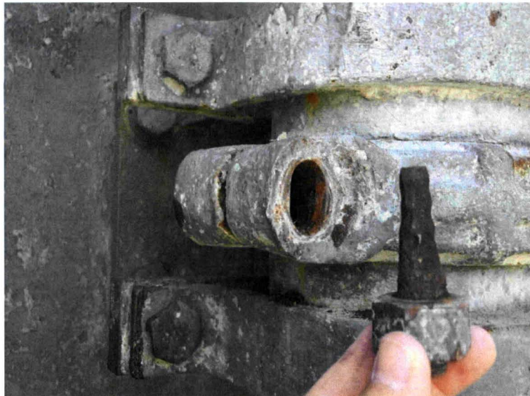
Figure 33. Pad 39B MLP-1: Bolt from Victaulic joint on center upper shield
