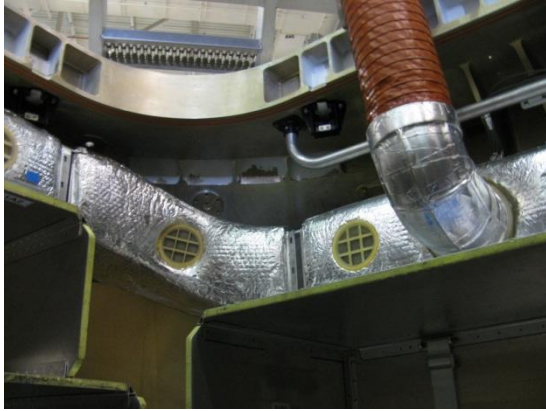
Figure 9. View of Duct with Inlet Vents Inside Dragon Pressure Section
