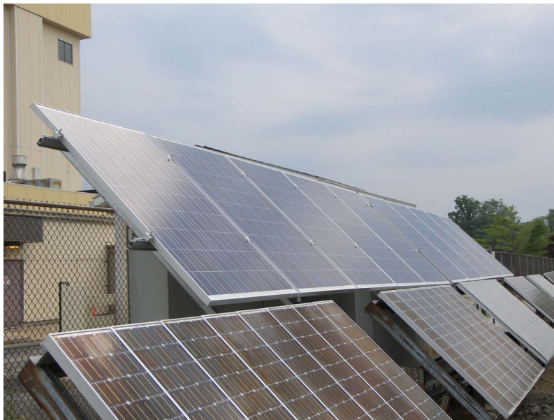
Figure 14.—A grid-tied photovoltaic system installed at GRC.
