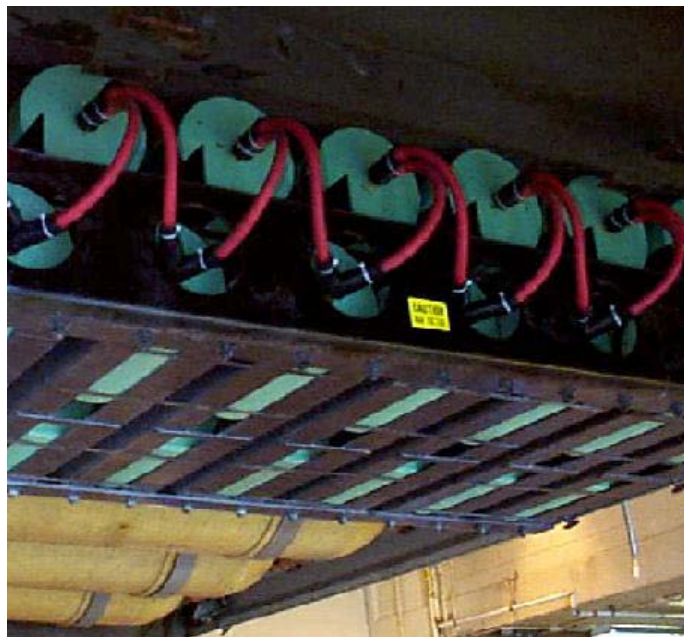
Figure 9.—The bank of ultracapacitors installed in the NASA Hybrid Electric Transit Bus (HETB).
