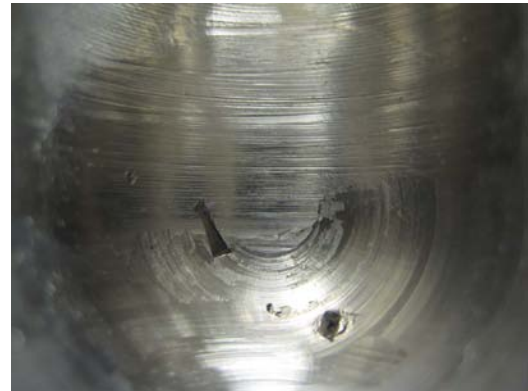
Figure X: GRC testing impact feature at 0.022” depth on first 90deg elbow downstream of FCV
