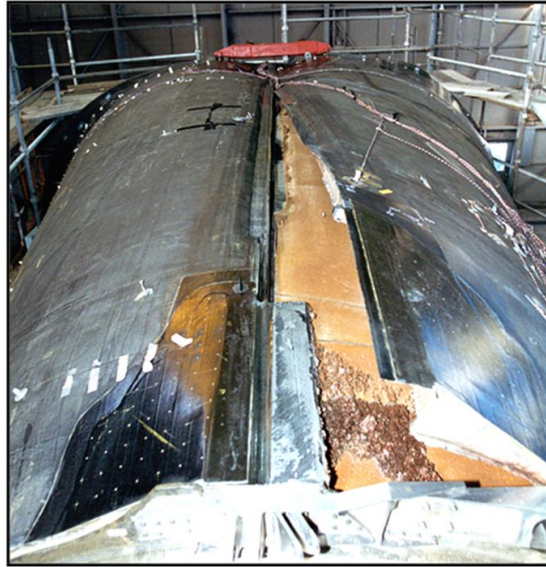
Figure 18-7. Failed X-33 Fuel Tank
