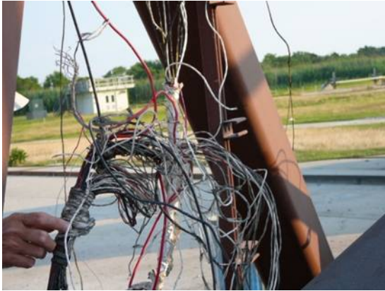
Fig. 12. Wiring damage, post launch.
