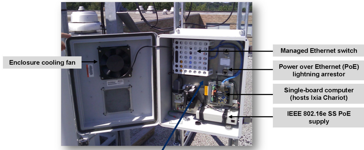
Figure 14.—Internal electronics of subscriber station (SS) enclosure.
