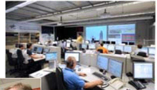
MUSC Ground Control Room
