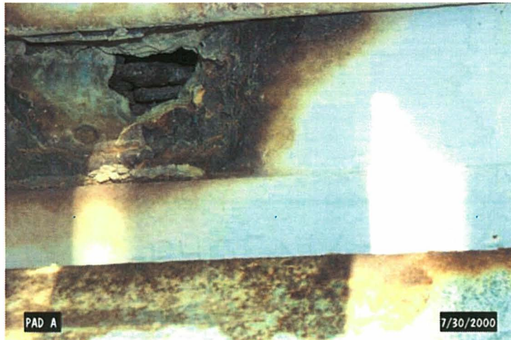
KSC Launch tower structural steel corrosion
