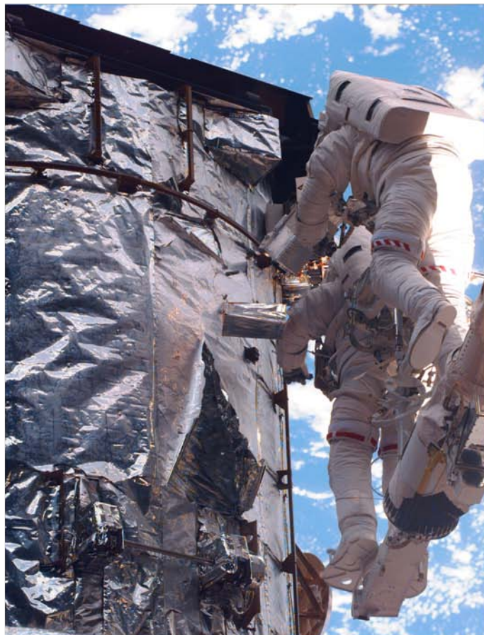
(c) Large radiation-induced cracks in multilayer insulation on HST as observed during Servicing Mission 2, after 6.8 years in space.[3]
