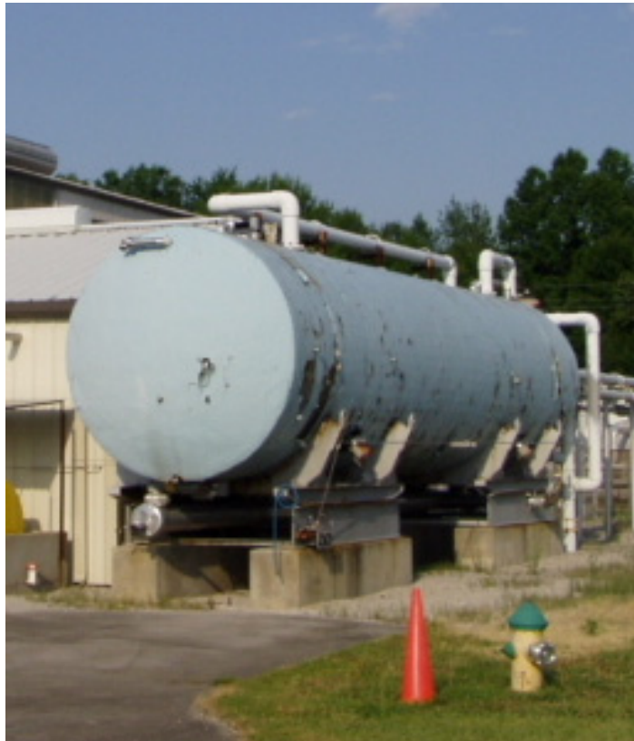
Figure 7.—Low pressure system cooling water supply tank (20,000 gal capacity).
