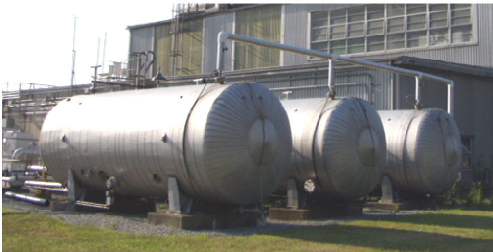
Figure 8.—High pressure system cooling water supply tanks (6000 gal each).
