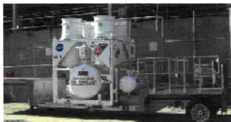
Figure 1. NASA/KSC Mobile Hydrazine Fuel Toxic Vapor Scrubber
