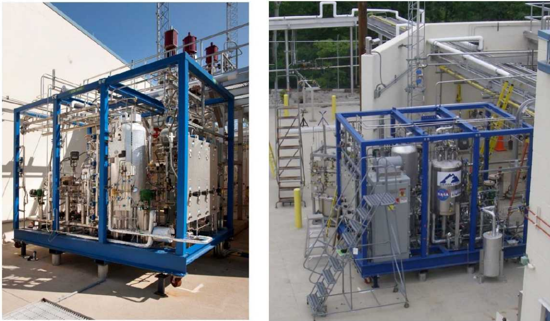
Figure 2: Photographs of LO 2 (left) and LCH 4 (right) PCFS Skids Outside of ACS
