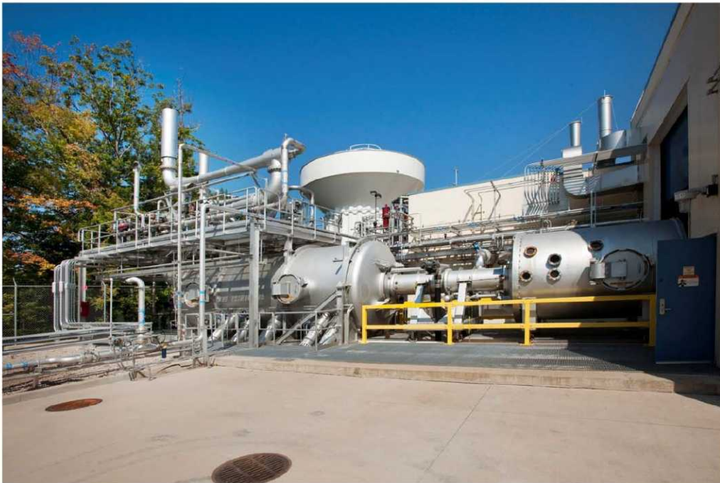
Figure 1: ACS Facility Test Capsule, Spray Cart and Ejector Platform
