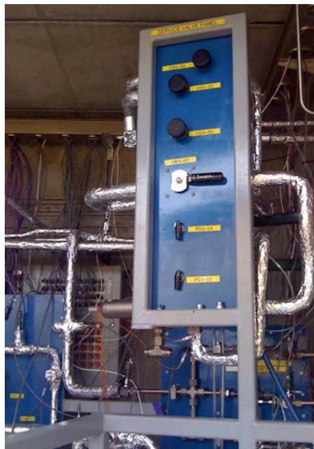
Figure 15. FS RoCS SDTA Service Valve Panel
