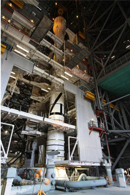
Figure 4. The Ares I-X first stage and new forward structures stacked in the Vehicle Assembly Building.
