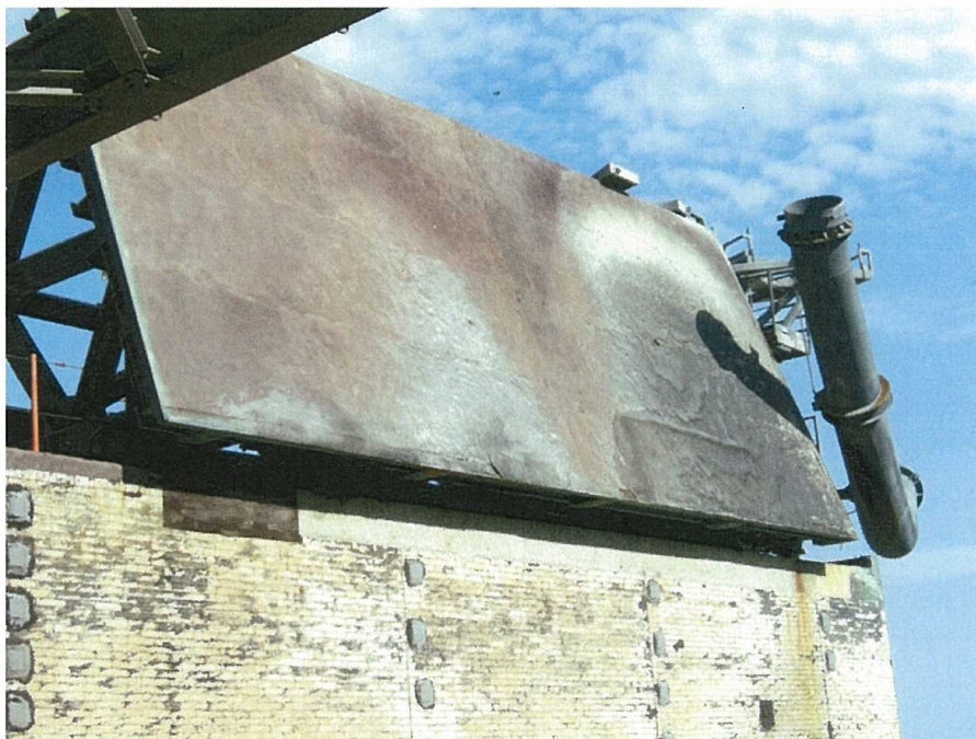
Figure 3. Side flame deflector.
