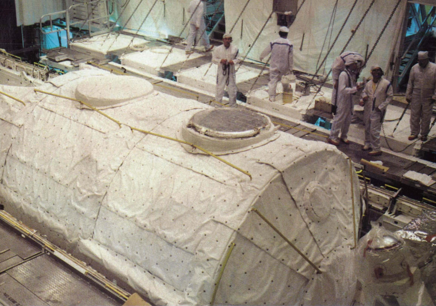
Technicians at KSC's Orbiter Processing Facility install Spacelab in the shuttle cargo bay.
