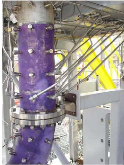
Figure 9. Water injection upstream of the elbow.
