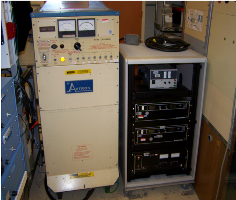
Figure 3.2.—Resistive load bank and power supplies.
