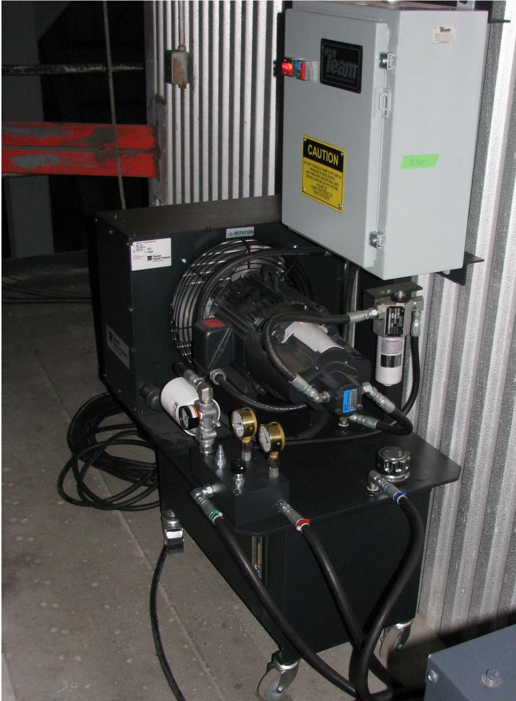
Figure 14. Hydraulic Power Supply.
