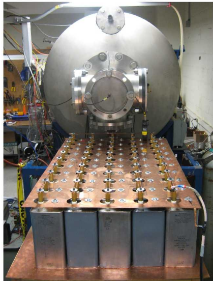
Figure 3. 3.2 kJ Pulse Forming Network and 1.5 m 3 vacuum tank.
