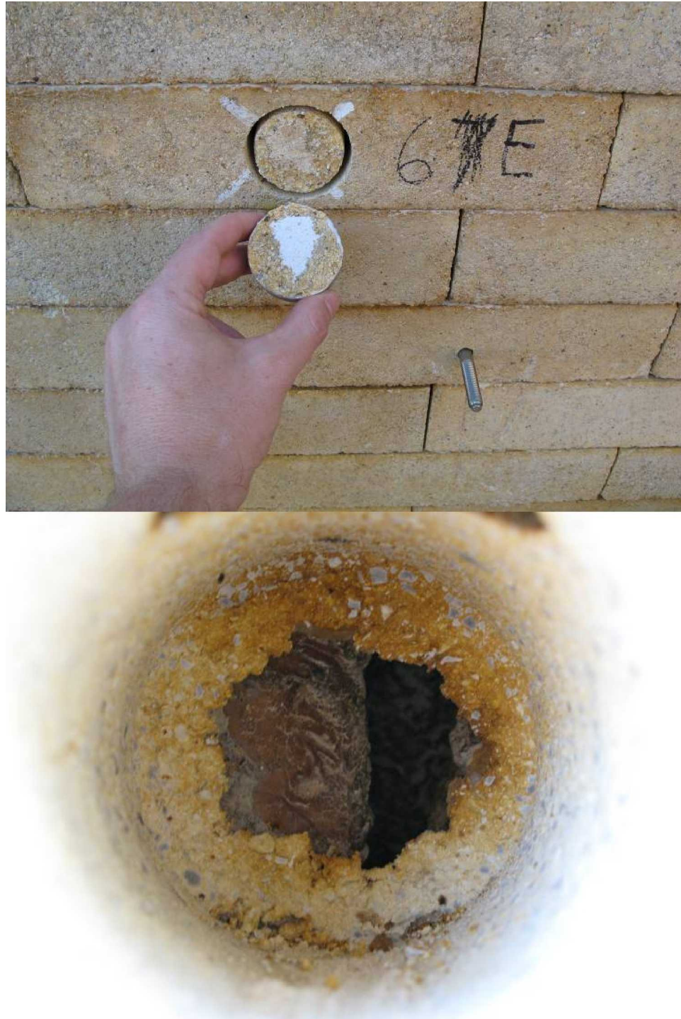
Figure 19. Core 6E – successful test: failed at 107 psi (image of pull stub and core face and the image inside the brick after the core was removed)
