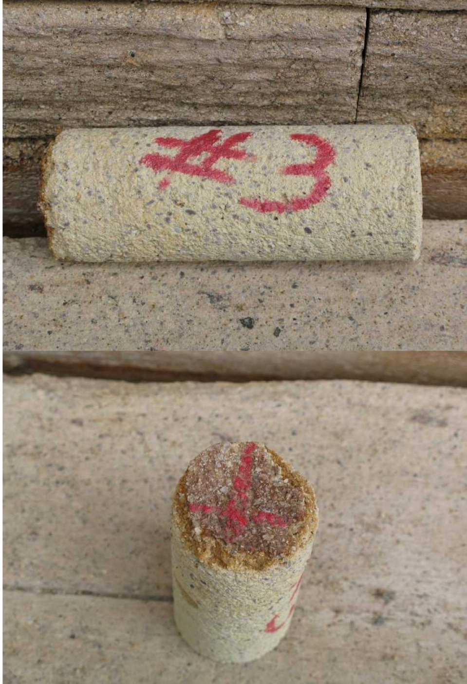
Figure 24. Core 3 – side image of core and outer surface of core removed during core drilling
