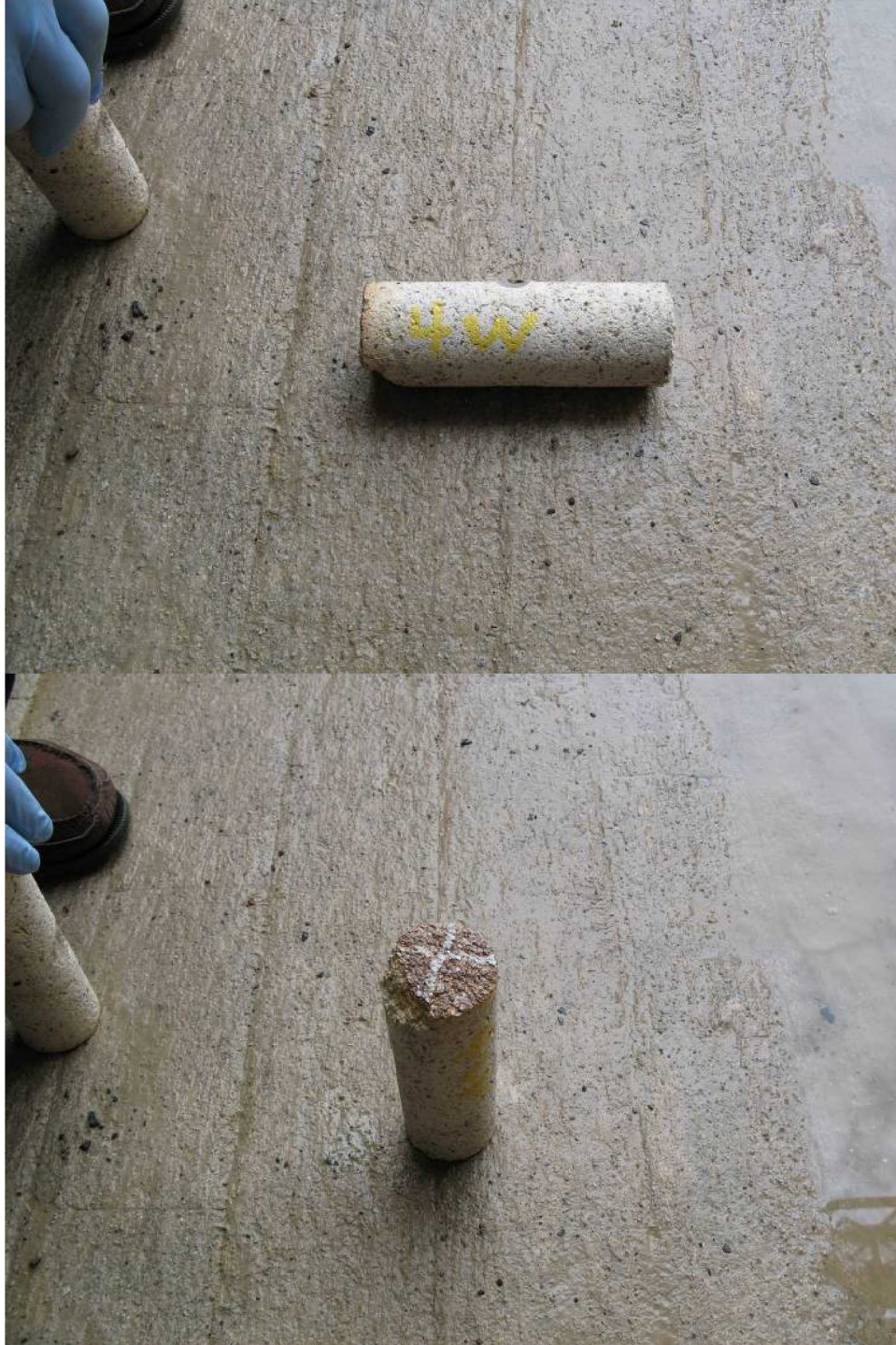
Figure 26. Core 4W – side image of core and outer surface of core removed during core drilling
