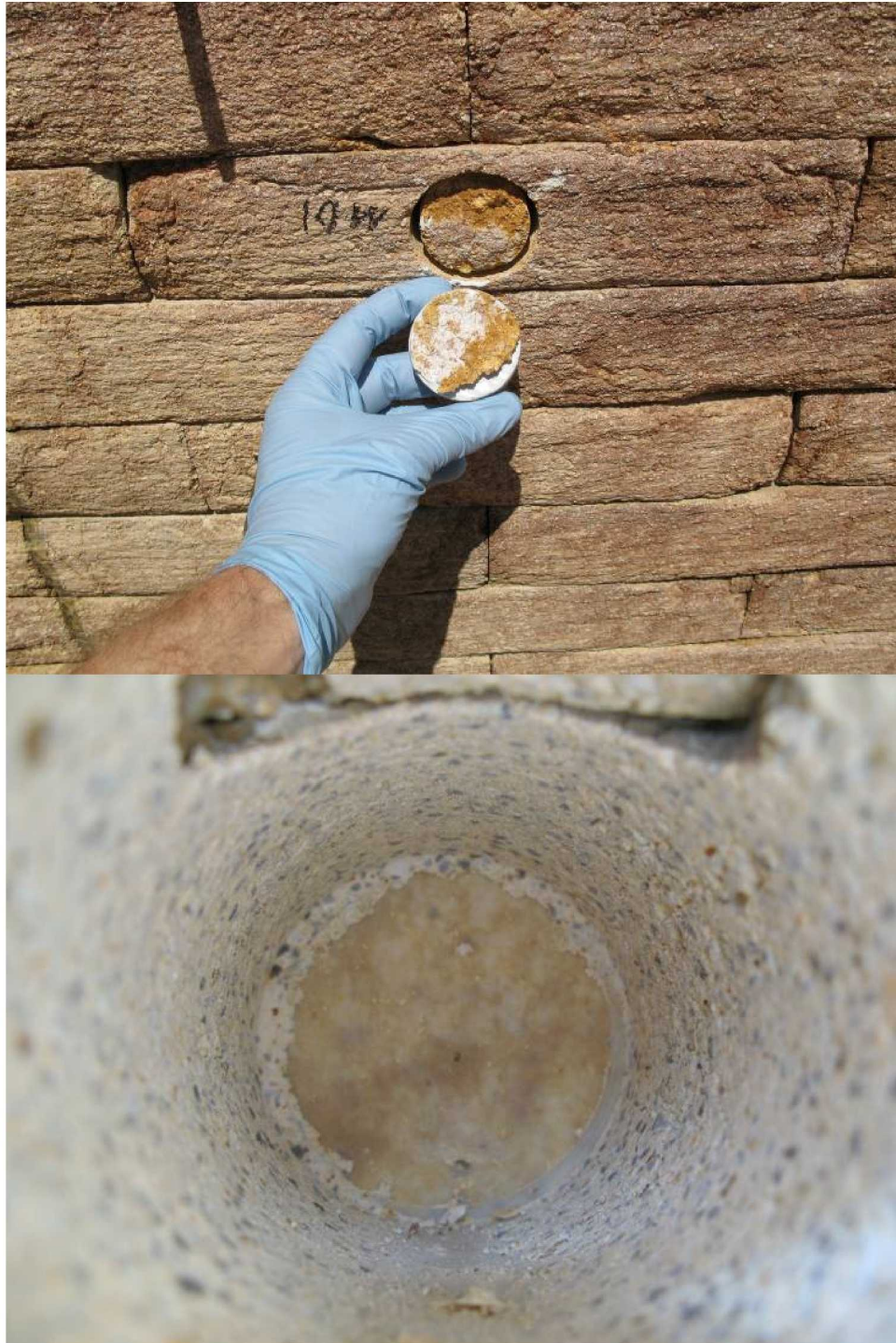
Figure 39. Core 10W – successful test: failed at 101 psi (pull stub and core face and inside the brick after the core was removed)
