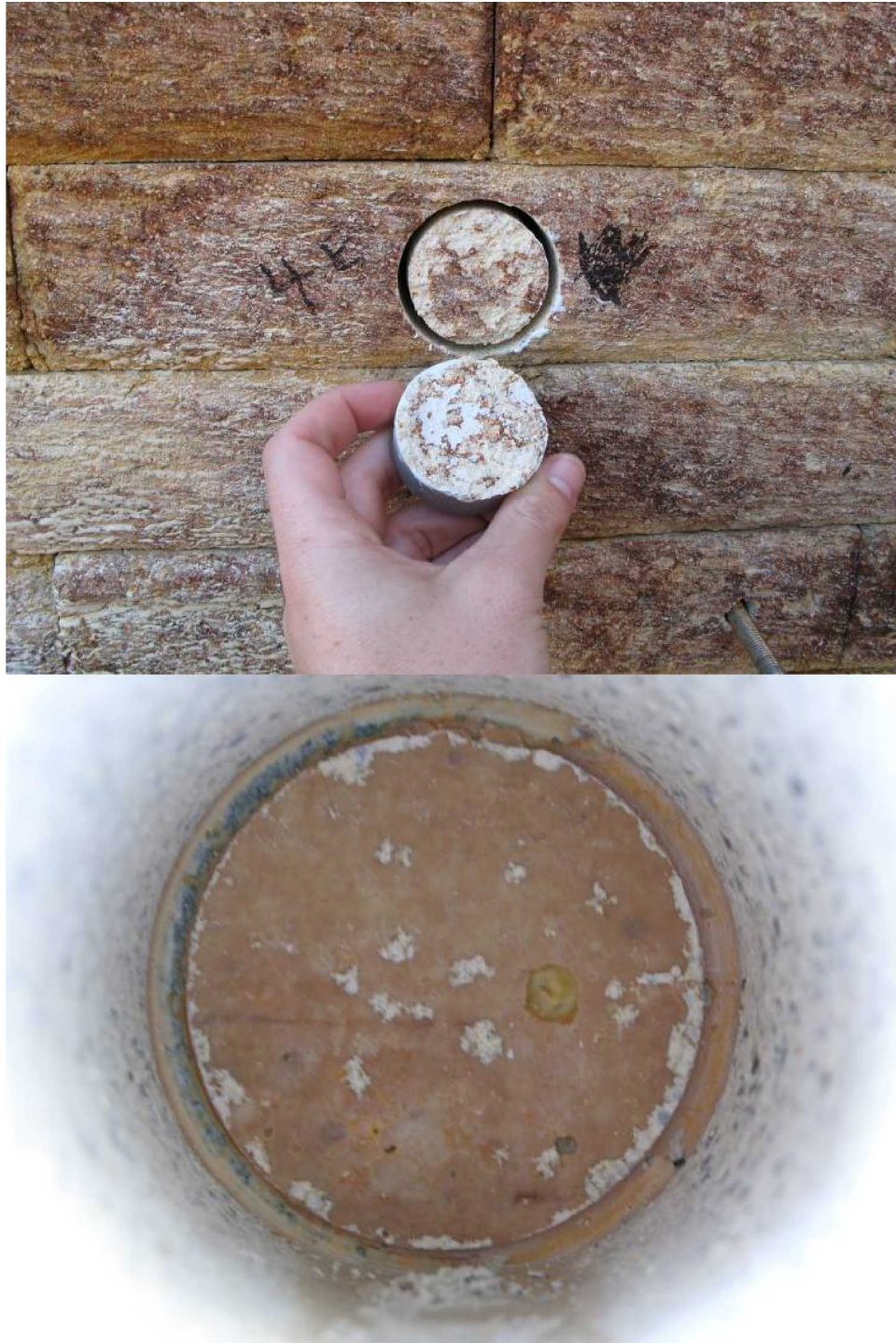
Figure 15. Core 4E – successful test: failed at 114 psi (pull stub and core face and the image inside the brick after the core was removed)
