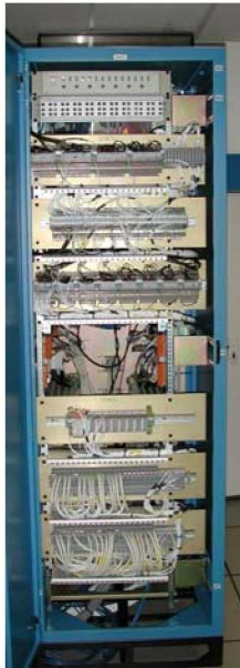
Figure 17. One of the Ground Command, Control, and Communication (GC3) racks, which will enable the Launch Control Center to communicate with and launch Ares I-X.
