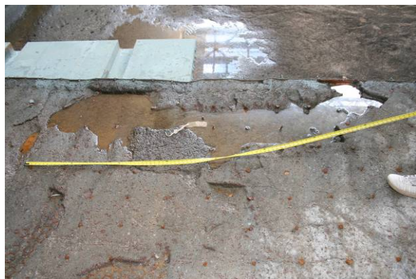
Figure 5. Location 3 shown in Figure 2(b): note spalling and heavy abrasion/erosion.
