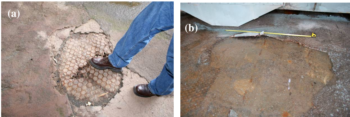
Figure 3. Location 1 shown in Figure 2(b): (a) prior to launch of STS-113; (b) after launch of STS-113 (note that spalled area has increased significantly).
