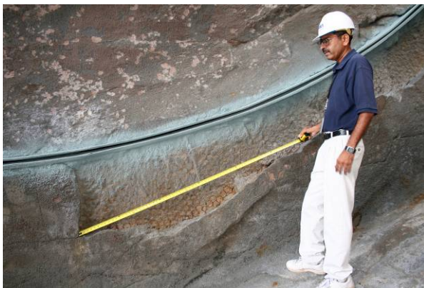
Figure 4. Location 2 shown in Figure 2(b): spalled refractory was approximately 4 inches thick.
