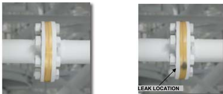
Figure 1. Irreversible hydrogen sensor before and after leak.
