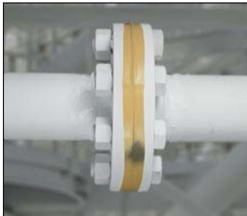
The dark spot on the "smart tape" indicates the location of hydrogen leak around this flange.
