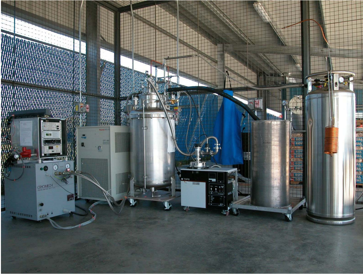
Figure 5. The densified hydrogen testing field facility at FSEC.
