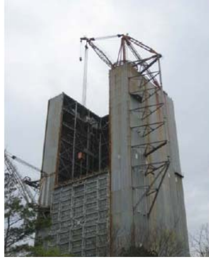
Figure 10. The side door was opened on Test Stand 4550 and the roof panels were removed for the first time in 29 years this past April.
