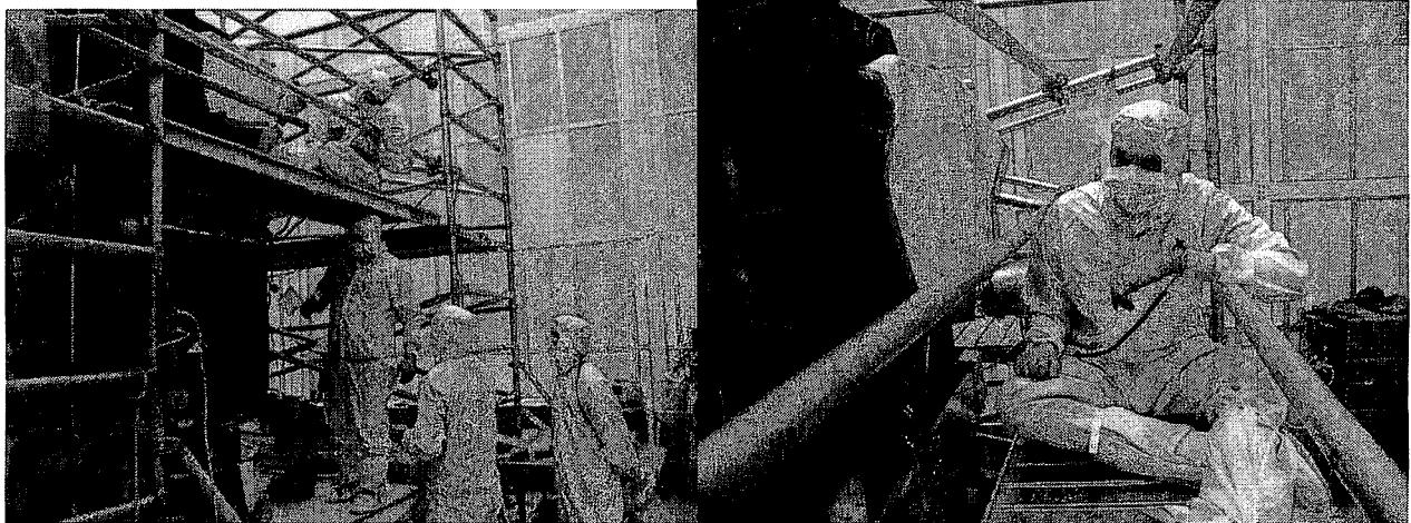
Figure 15 a) William "Joe" Thomes on second level scaffolding and Richard Chuska routing behind where HGAS will be stowed for launch, b) William Joe Thomes, performing FOB 3 routing on the early morning shift before space craft operational testing begins for the day.
