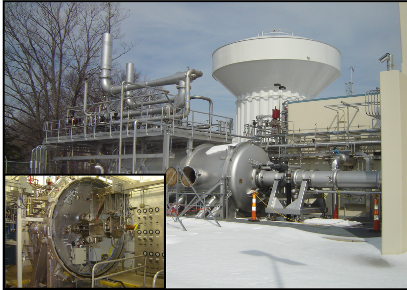
Figure 7. ACS facility at NASA-GRC
