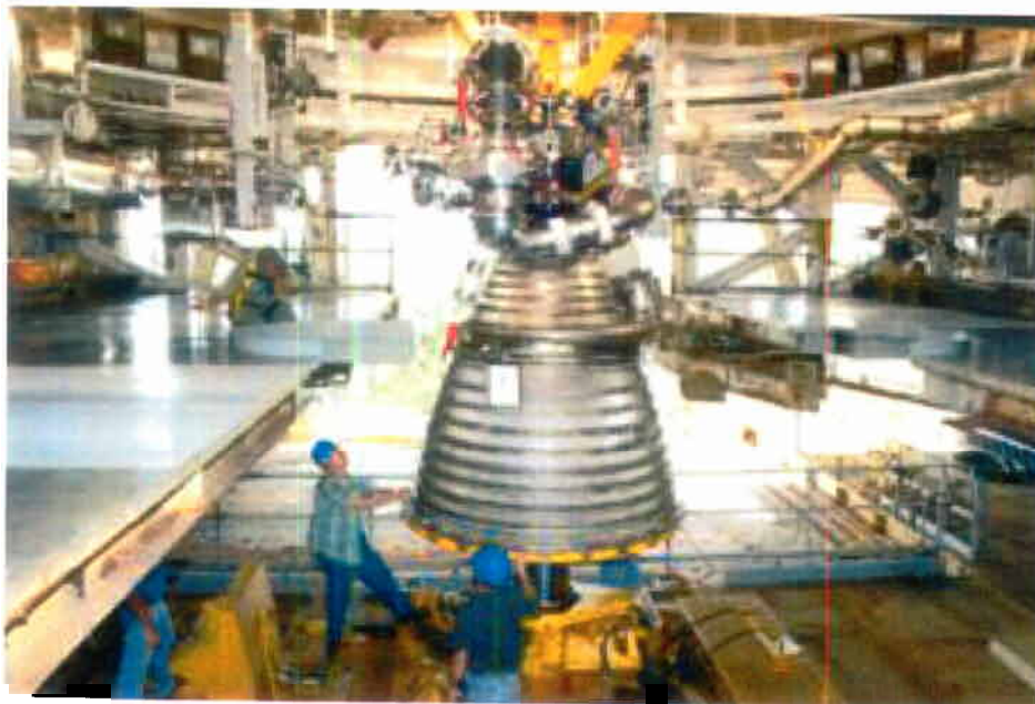
Figure 8. Installation of the heritage hardware powerpack in Test Stand A-1 at NASA SSC
