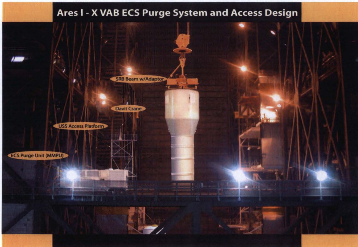
Figure 19. Changes made to the VAB for Ares I-X will be testing opportunities for regular Ares I stacking operations.
