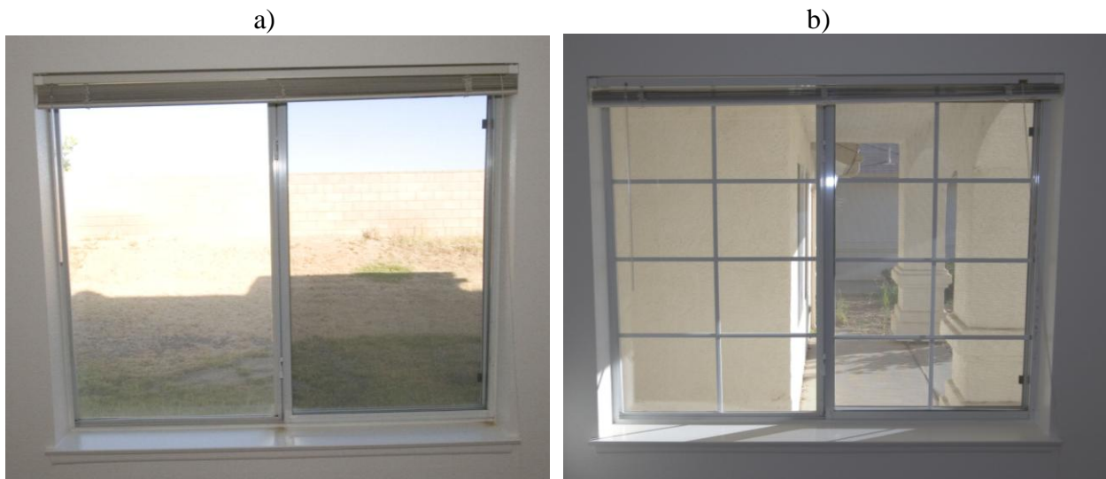
Figure 8: Photographs of the horizontal slider windows in a) the master bedroom and b) the front bedroom of the 2007 house. The right sash of the window is operable. The left is fixed.
