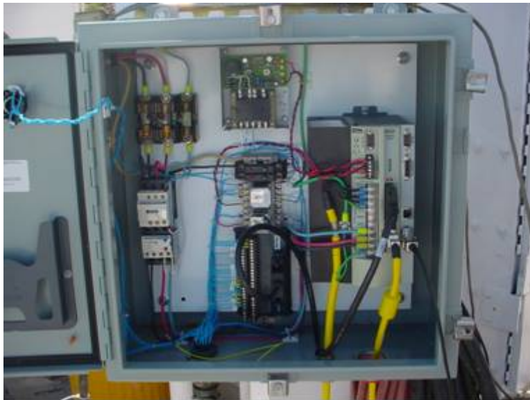
Figure 320. Electrical Assembly Of The Gemini Controller Box And The Remote Controller Panel Were Completed.
