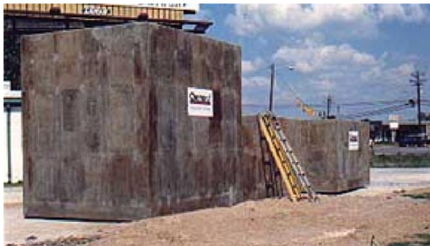
Figure 4. Precast Chempruf Sulfur Concrete tanks for Aqua Regia.
