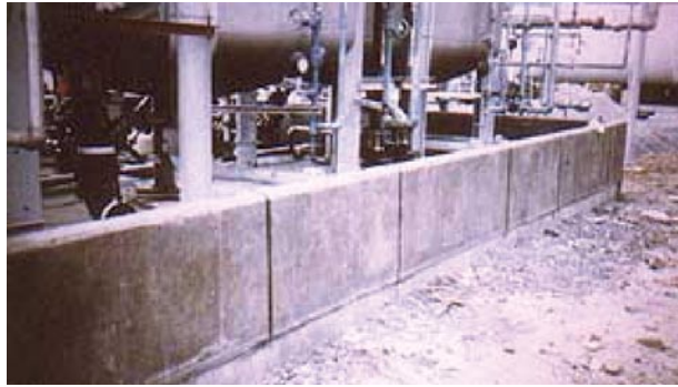
Figure 3. Chempruf Sulfur Concrete: acid containment system.
