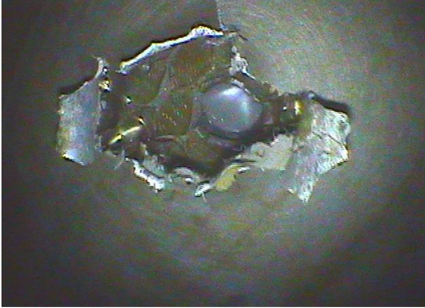
Figure 3: 12mm by 19mm hole in the rear facesheet of the radiator panel
