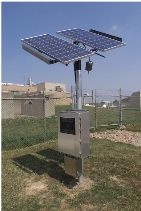
Figure 14.—An ultracapacitor backed photovoltaic power system at GRC.
