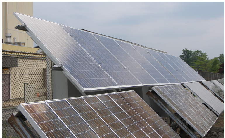
Figure 15.—A grid-tie photovoltaic system installed at GRC.
