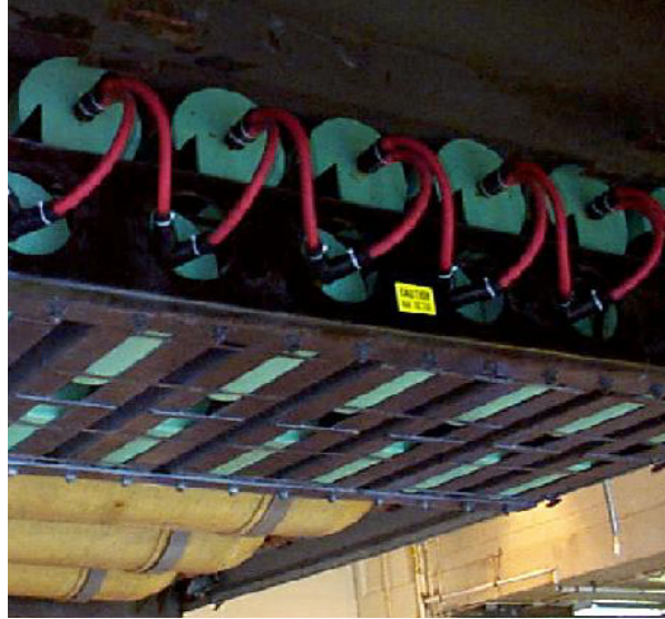
Figure 4.—The bank of 30 ultracapacitors installed on the NASA Hybrid Electric Transit Bus.
