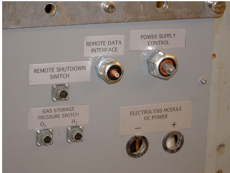
Figure 2.10.—OGP control system interface panel.
