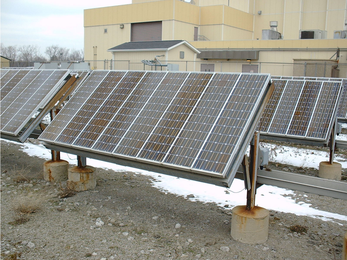
Figure 4.4.—Eight-panel sub array in the present array field.
