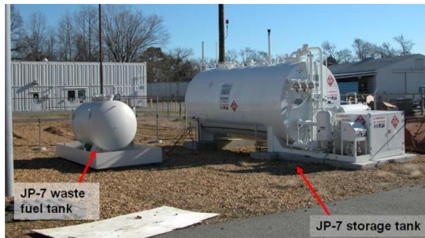
Figure 9. JP-7 Storage Tank and Waste Recovery Tank
