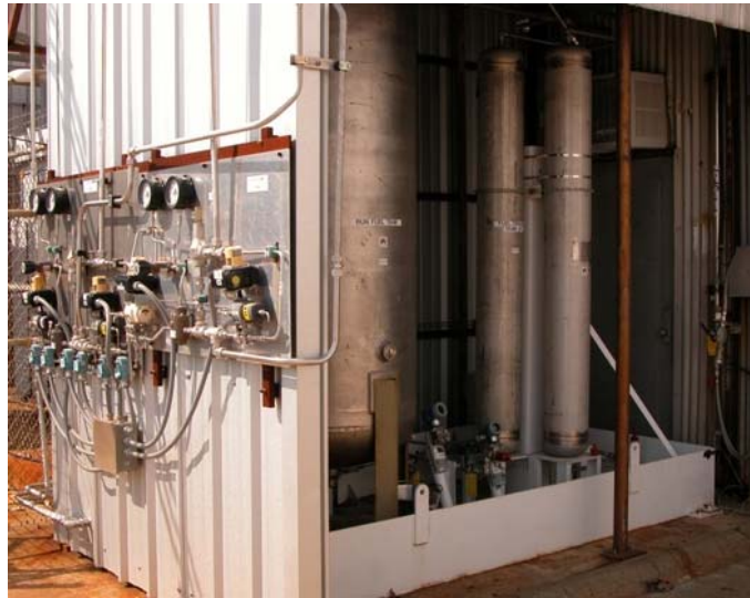
Figure 10. JP-7 Run Tank and Fueledraulic Tanks
