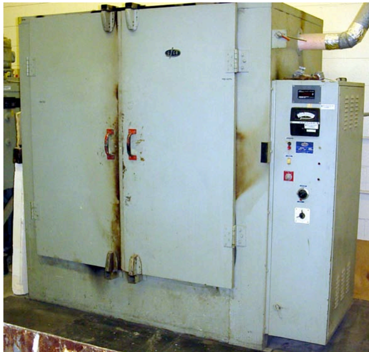
Figure 7. Curing oven for overnight firing investment molds to 550°F.
