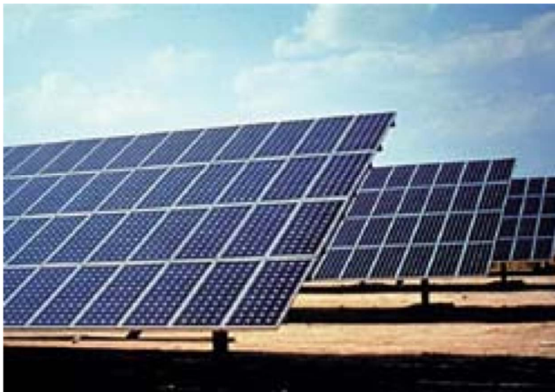
Figure 11.—Solar power station in Toledo, Spain (courtesy of BP Solar).
