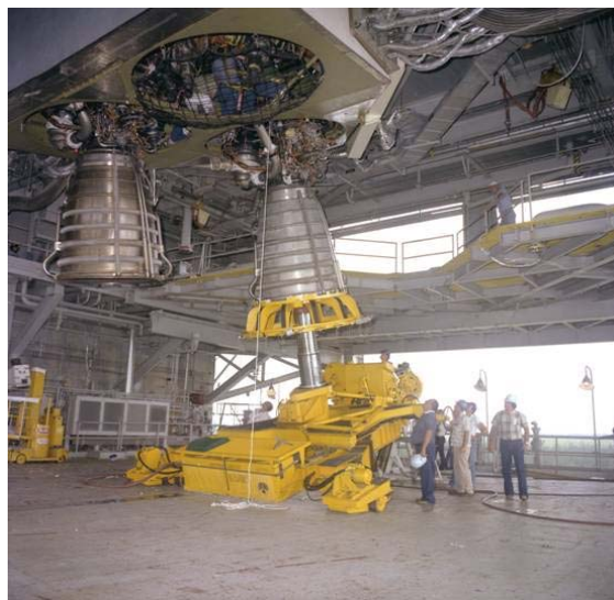
Figure 6. Installation of multiple SSME engines into housing for the MPTA stage test series.
