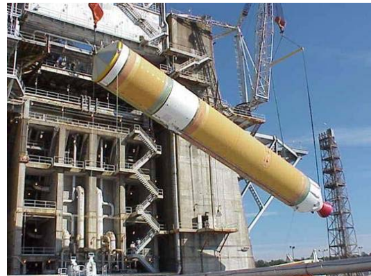
Figure 8. The Delta IV Common Booster Core is installed into B-2 test stand at SSC for stage test series (flight stage incorporating 1 RS-68 engine).
