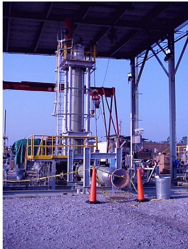
Figure 3. Hybrid sounding rocket (HYSR) test article installed at the E-3 Cell 1 test stand; solid fueled motor with liquid oxygen supply tank constitutes a simulated "stage."
