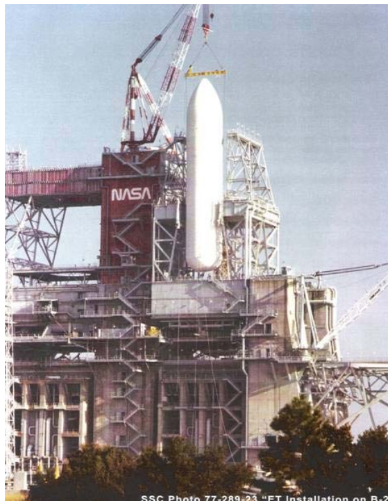
Figure 7. Installation of Shuttle ET into B-2 test stand at Stennis Space Center for MPTA stage test series (ET with 3 SSME engines).
