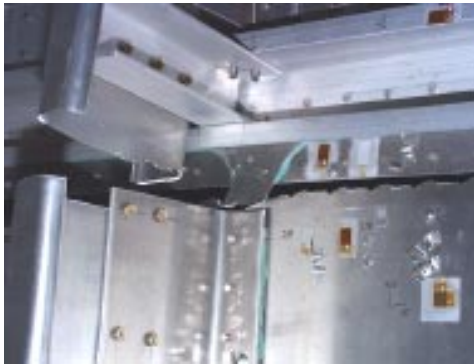
(b) Failed tear strap and frame
