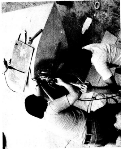
(e) Drilling pilot holes which will be enlarged to insert steel studs.
