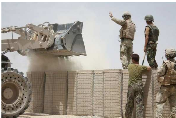
Fig. 1. Blast protection HESCO [9]
