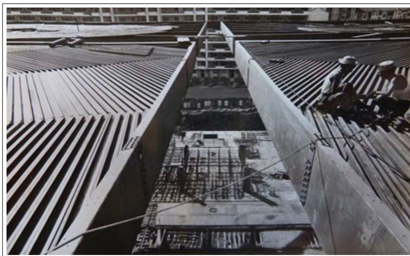
Figure 14: The Palace of Labour, the original roof in steel, removed in 1963. [Courtesy of PlannING]
