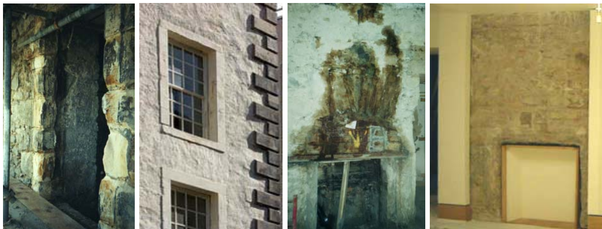
Figure 5. Before and after the works [a] External masonry and window margin [b] Internal wall and fireplace
