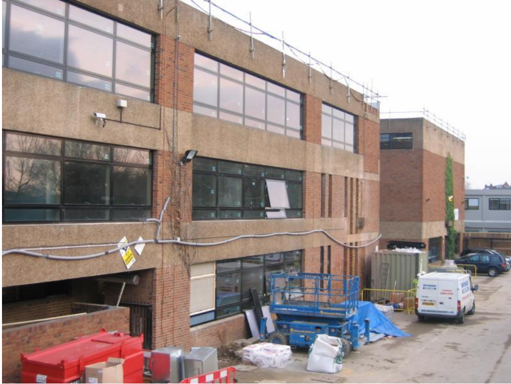
Photo 5.6 The existing buildings at Eastwick Field: it was decided to retain most of these, in spite of problems with disabled access
