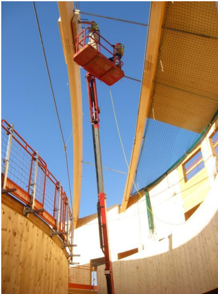
Photo 6.8 The offsite fabrication and an innovative edge support system, shown here, obviated the need for scaffolding and greatly improved access during construction.
