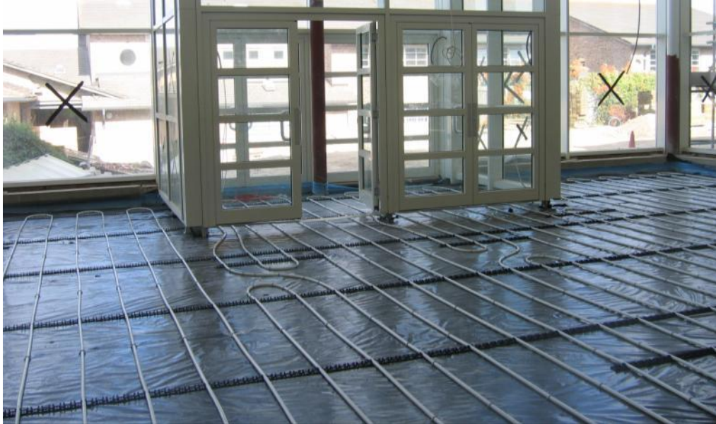
Photo 5.1 Underfloor heating pipes being laid in new atrium, connected to ground source heat pump
