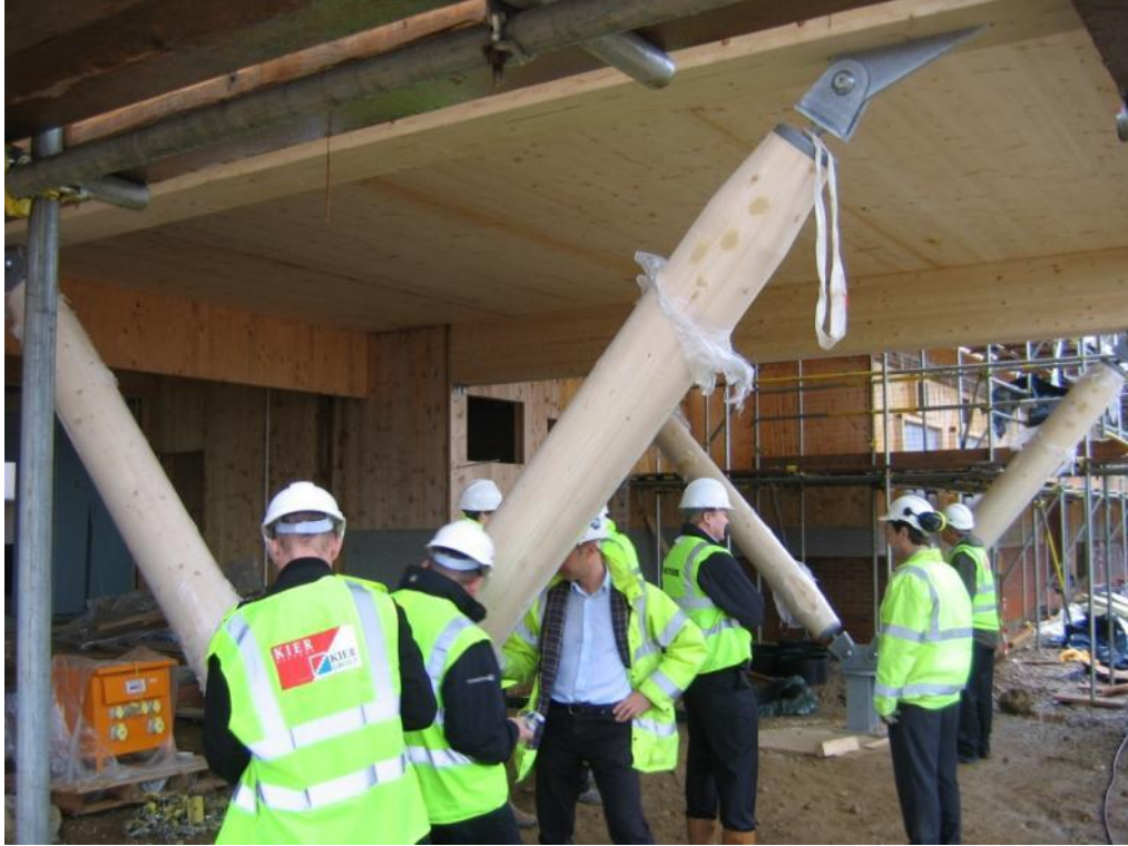
Photo 6.2 The timber system led to considerable interest and frequent visitors to site. This group included a potential school client and architect for a project which was later won using the same system.
